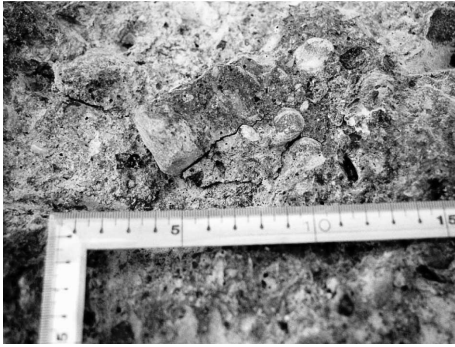
Fig.9 Cracks on the treated surface by handbreaker.
