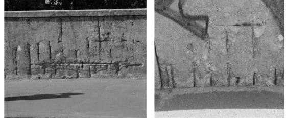
Fig.2 Deterioration is caused by carbonation.
