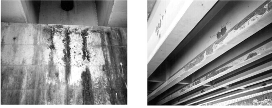
Fig.1 Chloride induced deterioration.
